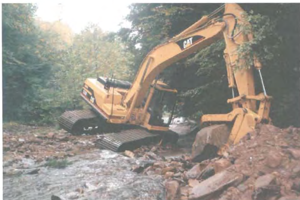
Figure E. The stream bottom was disturbed by the construction process.
