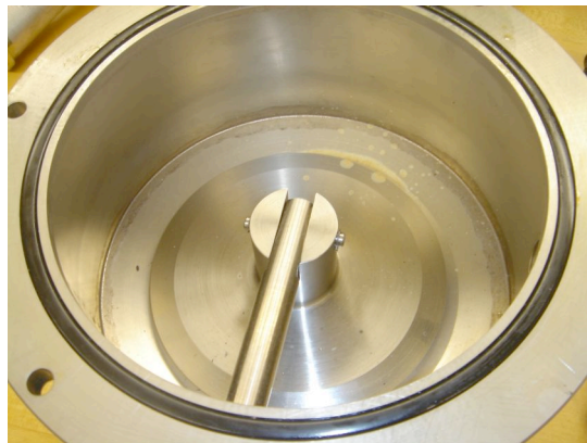
[Fig. 6b]: Closed baffle valve to terminate diffusion pumping.
